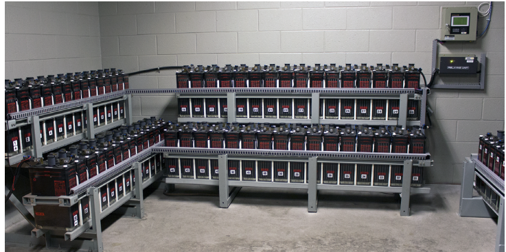
iPQMS Installation on 125VDC Utility Battery System
